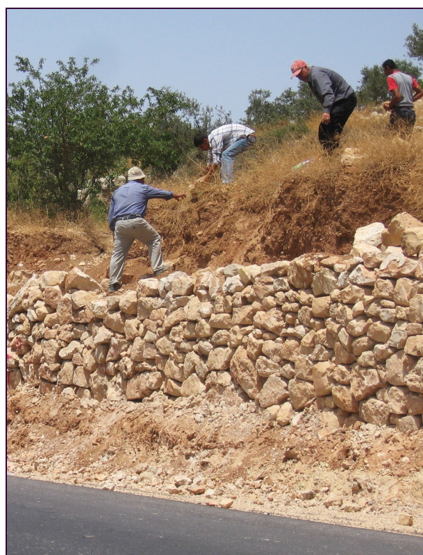
Photo: Ancel Kats/WFP—Food-for-Work site in Halhul village, Hebron Governorate, 1 July 2009 — Building of retaining walls on a newly built agricultural road [with USAID funds] connecting two villages .
